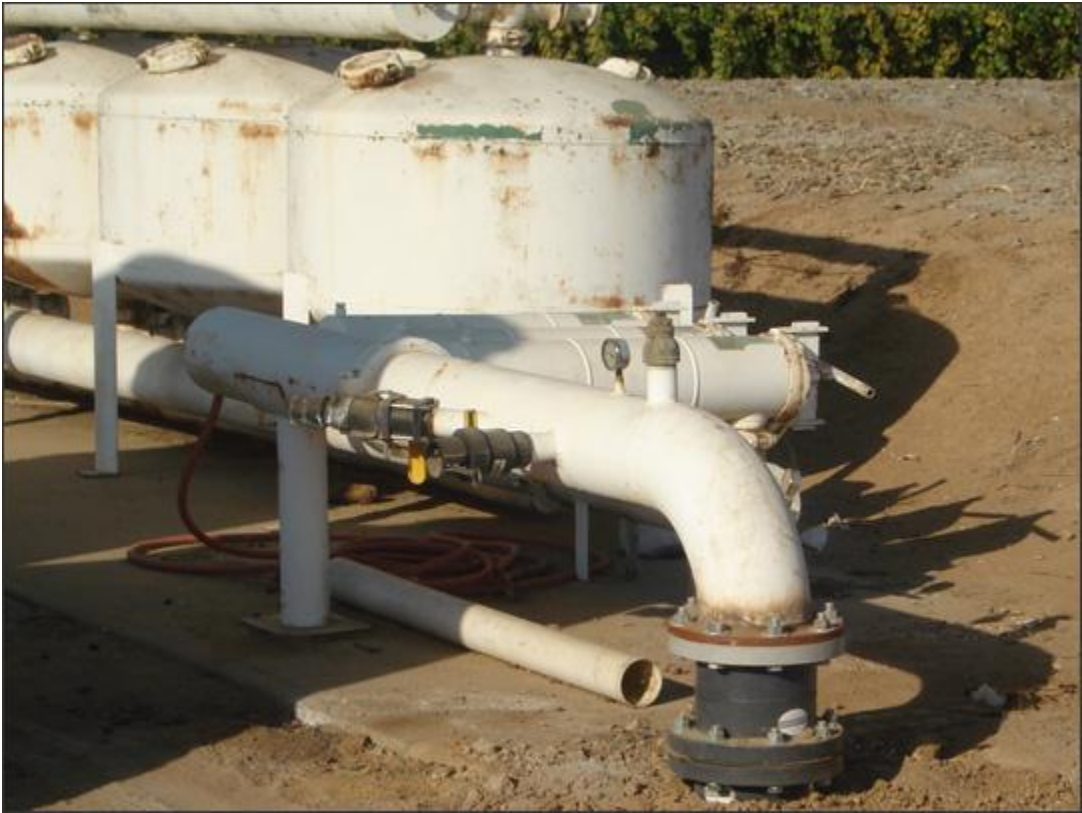
10" H2O ENERGIZER Ag System installed at pump after filtration:
