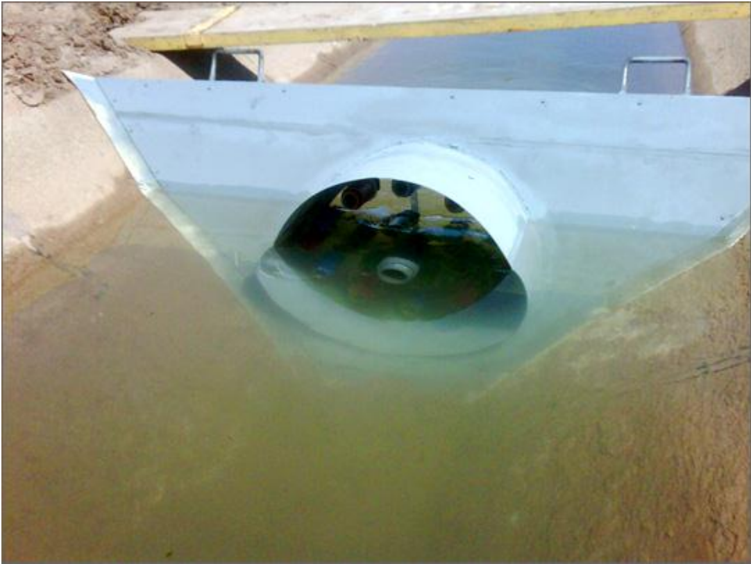
24" H2O ENERGIZER Ag System installed in flood/ditch irrigation:
